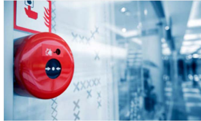
Fire Protection System
